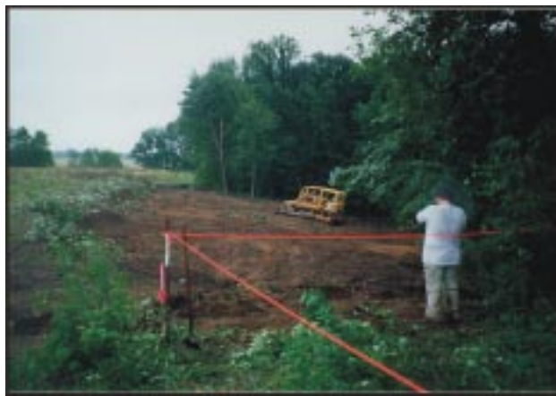
MVAC's Jon Baker protects the conical mounds of the Eagle Group during construction.
